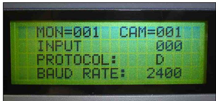
LCD of keypad CCT786 & CCT768 with correct default setting for this dome at address 1
