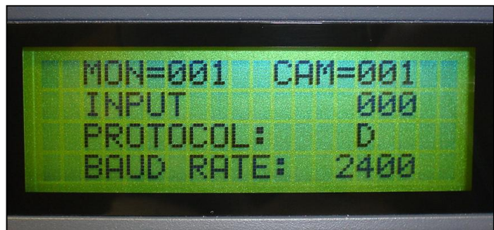
LCD of keypad CCT786 & CCT768 with correct default setting for this dome at address 1
